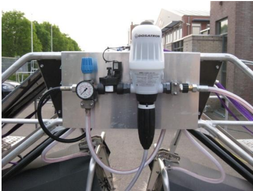
Img. 37 Dosage pump for cleaning compound
